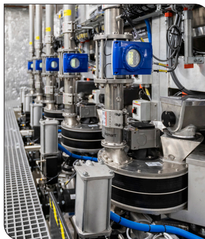
Illustration 3: Water meters installed on several WBF's
